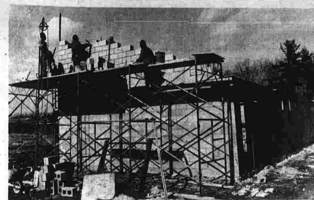
Band shell taking shape. The Bicentennial band shell, located on the campus of Manchester Community College, is taking shape and if the weather holds out the block work will be completed this week, according to Joseph Swenson, contractor for the work.
